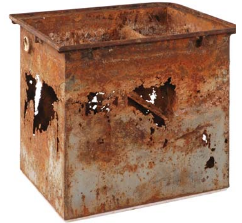
Corroded Wet Inlet Grease Interceptor
