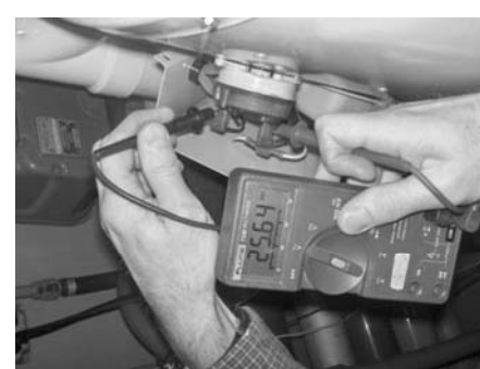
Checking pressure switch contacts. Contacts are open if blower is operating and there is 22-26 volts measured between the two contacts (as in photos)
