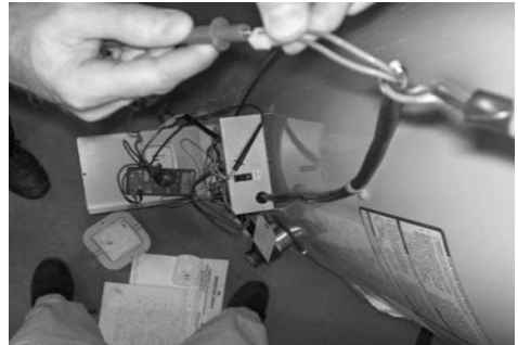
Checking continuity of upper sensor wire harness.
