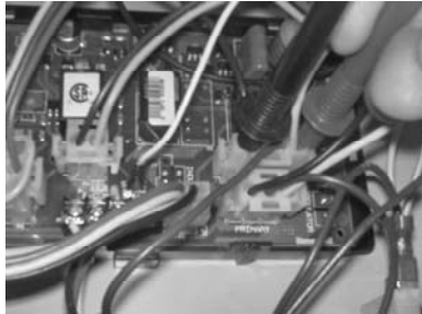
Checking line voltage to board. Pins to black and white wires.
